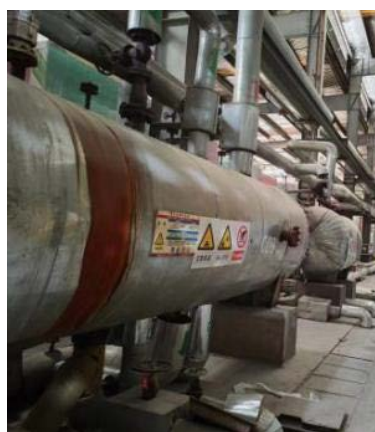
Figure 3. Steam flash tank
