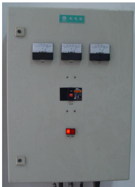
Figure 2. Radar distribution box
