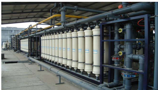
Figure 3. Organic ultrafiltration membrane process for wastewater treatment 图 3. 有机超滤膜处理废水工艺
