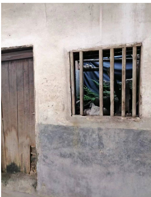
Figure 8. Wall damage in Dongshan Academy 图 8. 东山书院墙体破损
