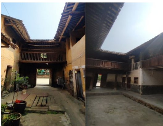
Figure 7. Wall damage of residents in Fuluji 图 7. 福禄炭居民墙体破损
