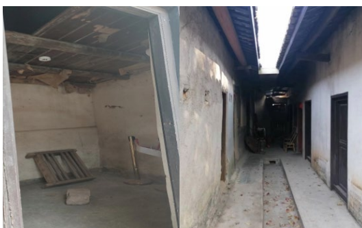
Figure 5. Wall damage in Lin Fengmian's former residence
