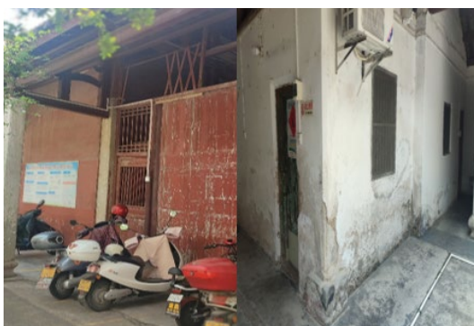
Figure 6. Wall damage of Dajue Temple
